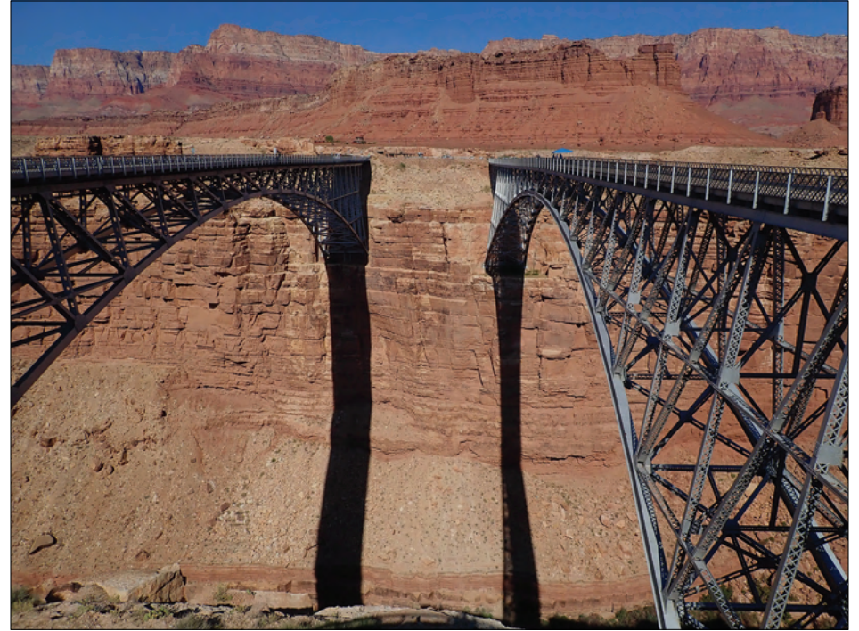
The two Navajo Bridges spanning Marble Canyon that are similar in appearance. The historic bridge, almost 100 years old, is on the right.
